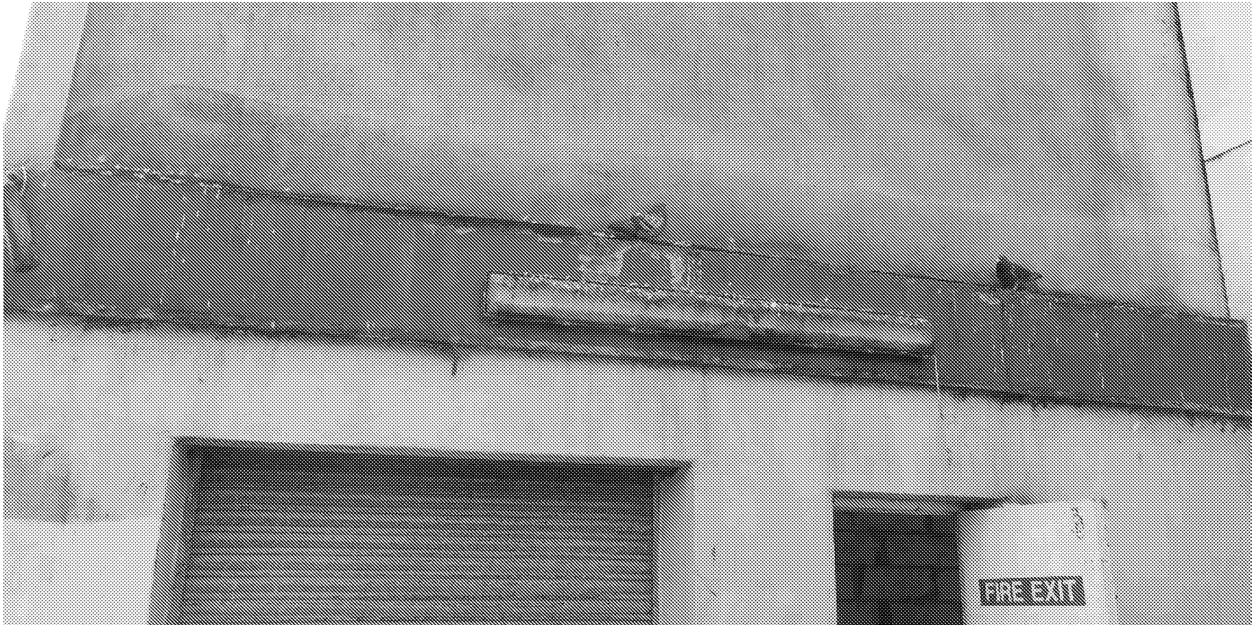
Image 20 -- External view: Note horizontal cracking above blue encasement
