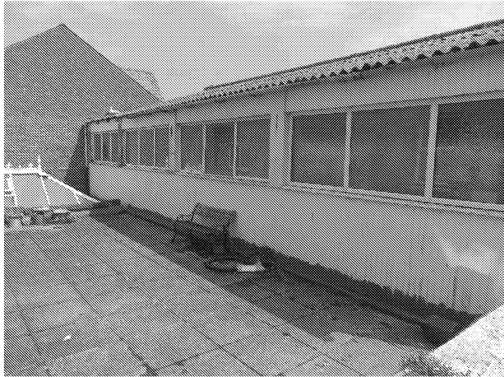
Image 10 – Asbestos roof sheeting and decaying timber boarding allowing water to seep through to primary beam below. Image 1 & 2 show the steel beam under
