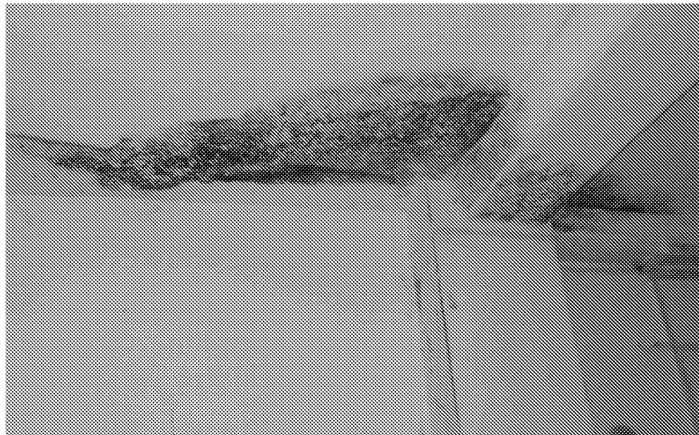
Image 12 – Mould created by water ingress from above
