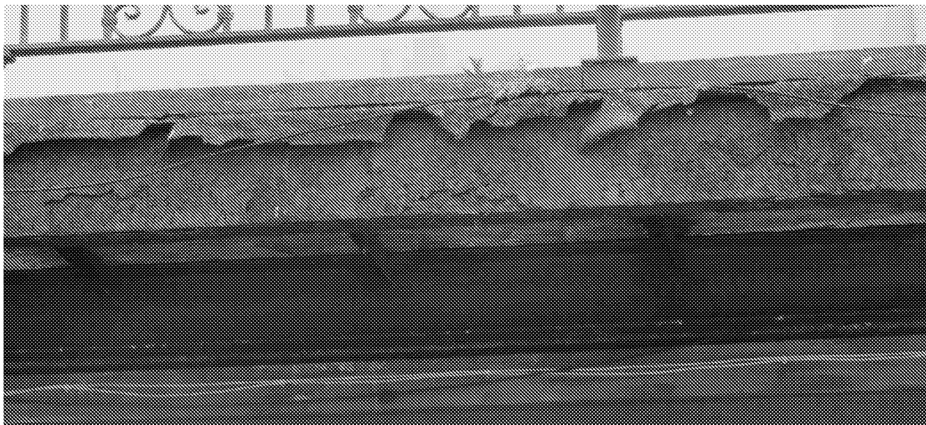
Image 5 - Waterloo Square Elevation – Severely laminated balcony steelwork at First Floor
