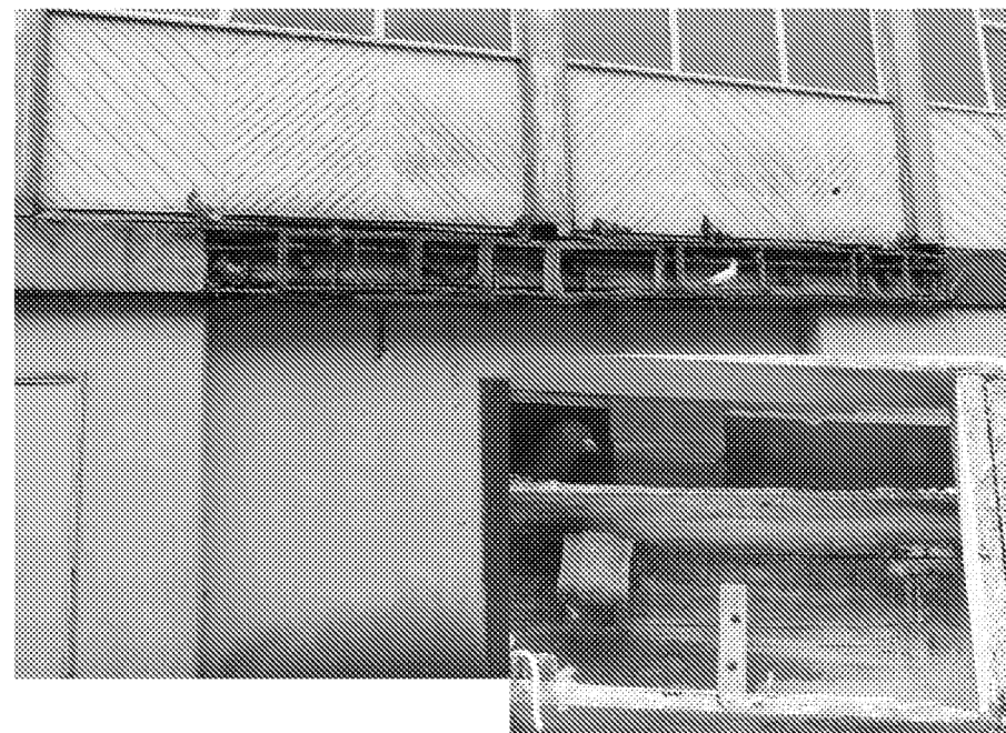
Image 4 – Primary beam supporting rear of first floor gym area Note the decayed timber and corroding steel beam Beam in Norfolk Street at ground Floor (Badly decayed timber boxing hiding a Steel Riveted beam)
