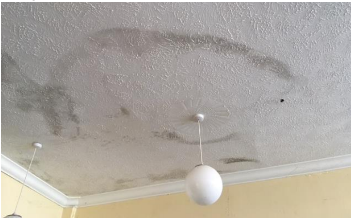
Image 13 – Water Ingress on upper Floors
