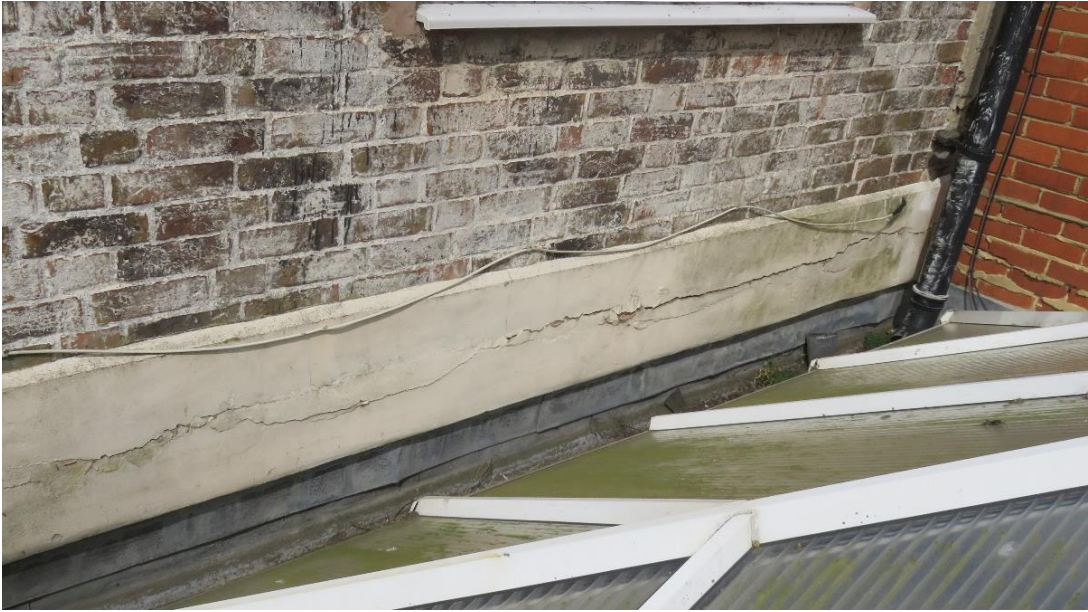
Image 3 - Severe cracking to render over support beams at First Floor (no safe access to investigate further) This is the opposite end of the roof lantern. Clearly the beam hidden by the render is corroding, hence the cracking
