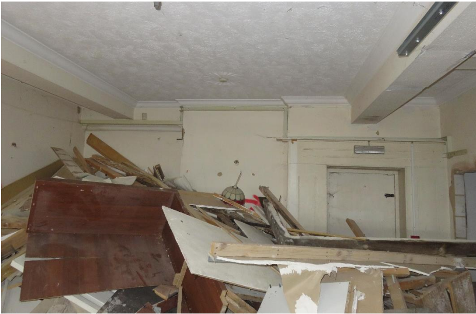
Image 11 – Extensive debris from previous abandoned refurbishment Hiding unknown Issues
