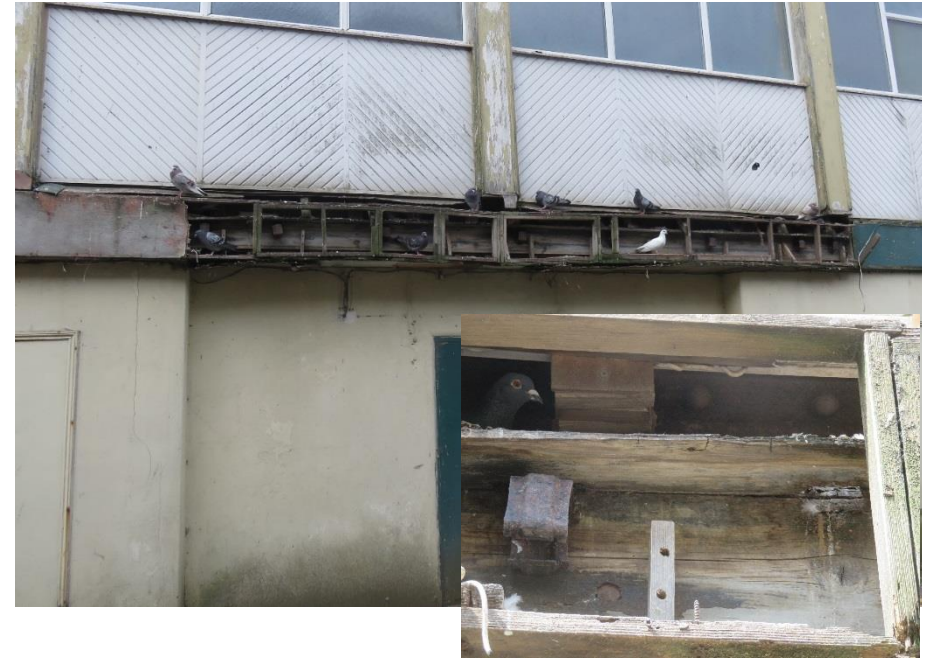
Image 4 – Primary beam supporting rear of first floor gym area Note the decayed timber and corroding steel beam Beam in Norfolk Street at ground Floor (Badly decayed timber boxing hiding a Steel Riveted beam)
