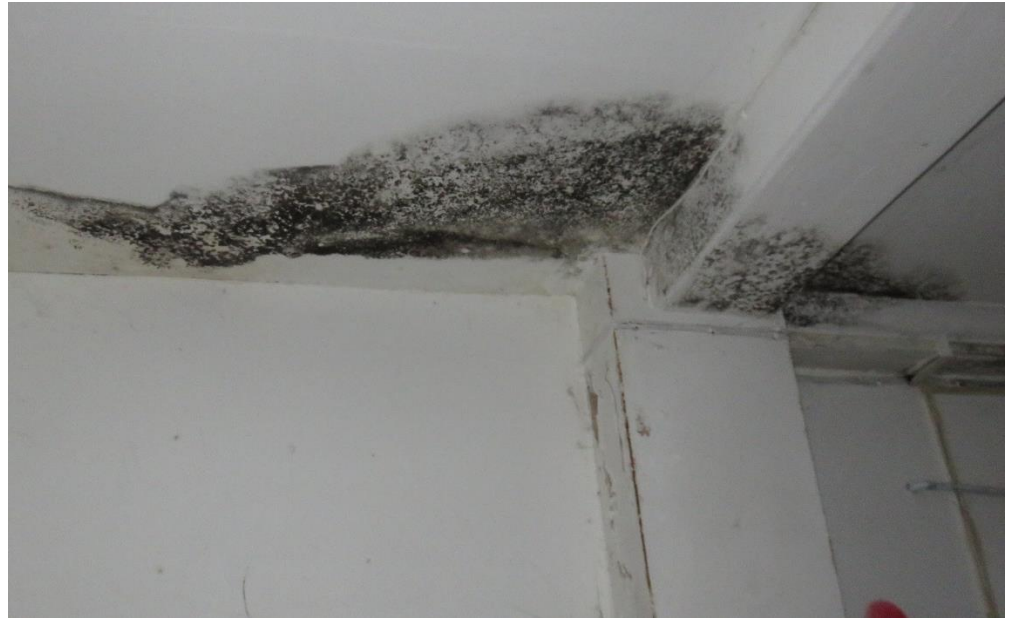
Image 12 – Mould created by water ingress from above
