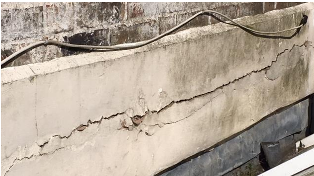
Close up of cracking to external structural beam protection
