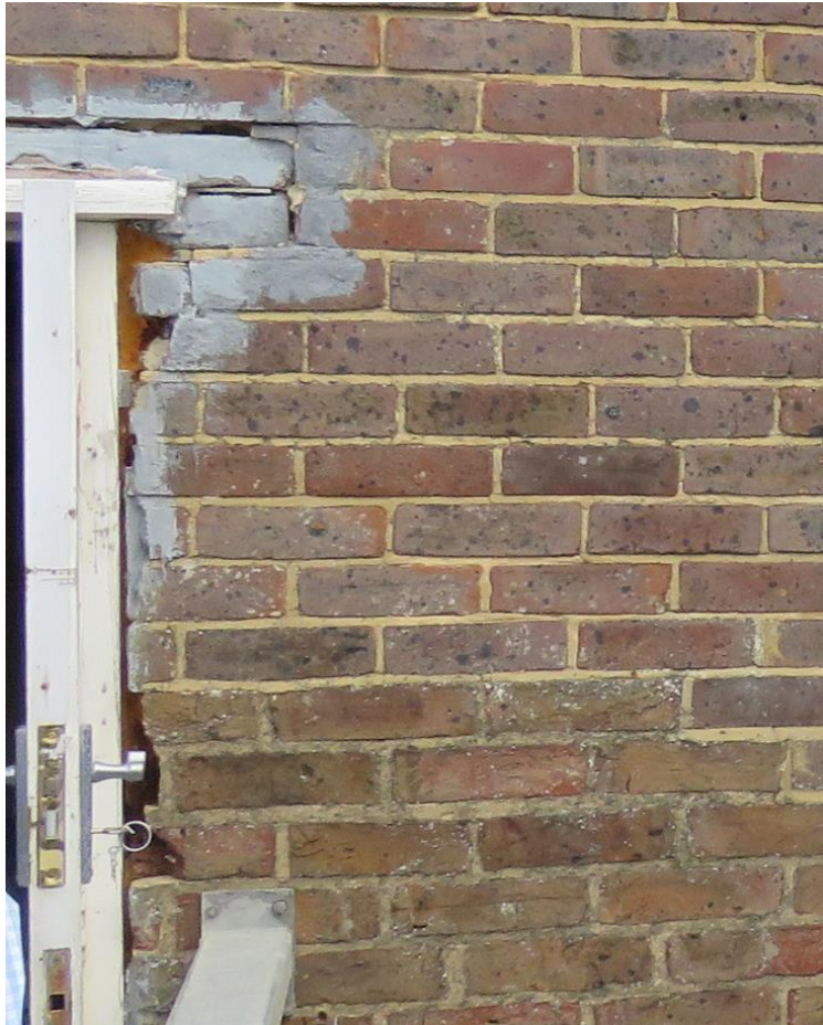
Image 9 – Poor construction works resulting in water ingress to steel supports below
