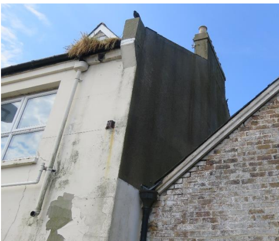
P11 – Cracking to 2 nd Floor rear elevation
