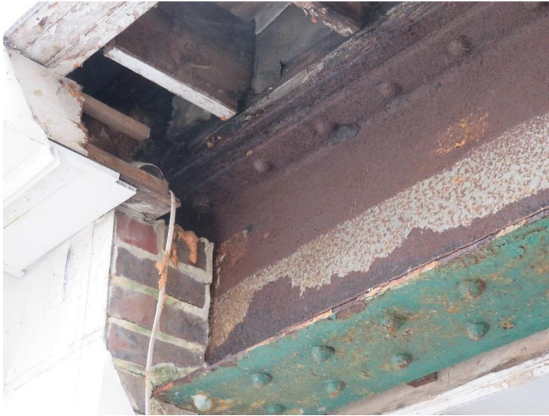
P12 – Internal Beam supporting Gym at 1 st Floor (note delamination of Bottom Flange)
