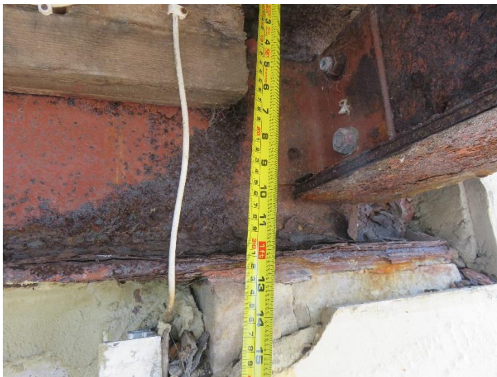
P13 – External beam (RHS) No. 2 Waterloo Sq Elevation (note delamination of Bottom Flange)
