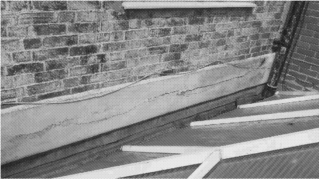
Severe cracking to render over support beams at First Floor (no safe access to investigate further)
