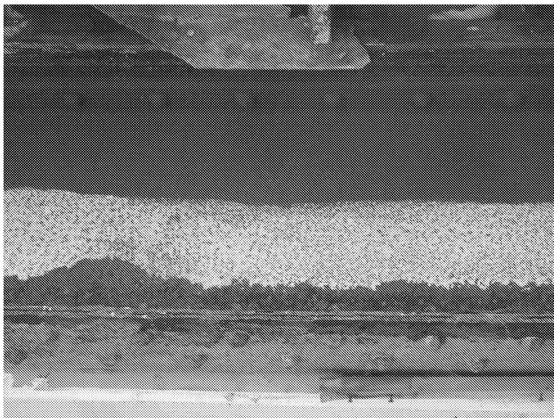
Primary Support Beam, supporting the floor and structure to the Boxing Facility (Viewed from Ground Floor) Note the lamination of the top and bottom metal plates and the extensive corrosion of the main beams web at the base of the beam.
