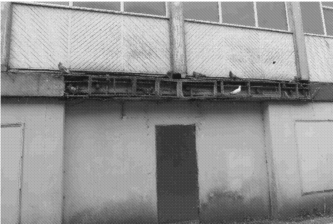
Beam in Norfolk Street at ground Floor (Badly decayed timber boxing hiding a Steel Riveted beam)
