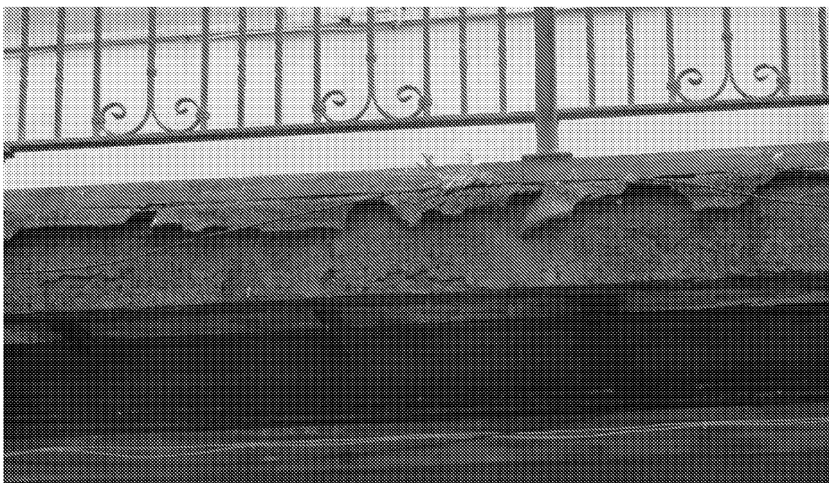
Waterloo Square Elevation – Severely laminated balcony steelwork at First Floor
