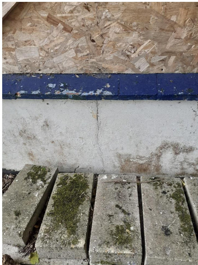
Crack in front elevation
