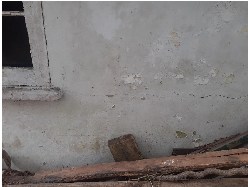
Cracking in garage East Elevation
