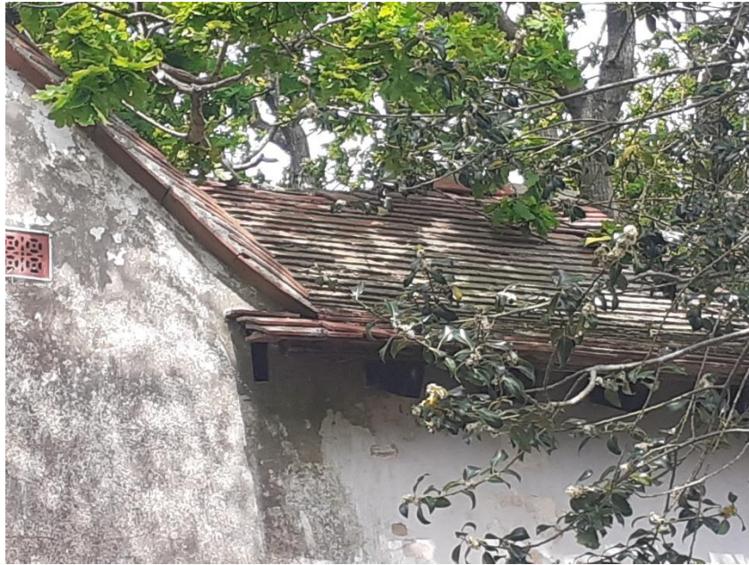
Roof damage from Oak
