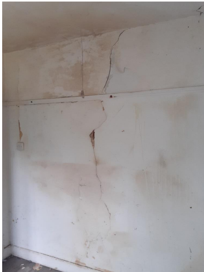
Cracking in rear bedroom
