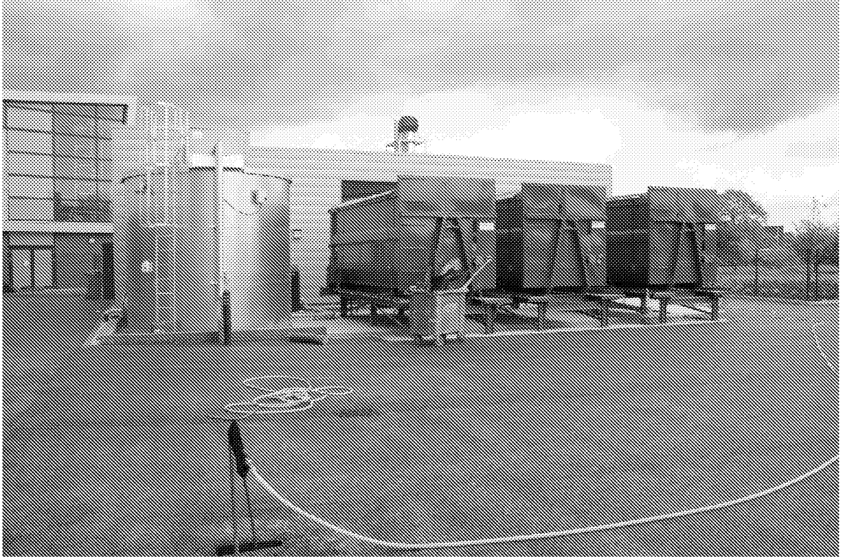
Close up from within the energy centre compound
