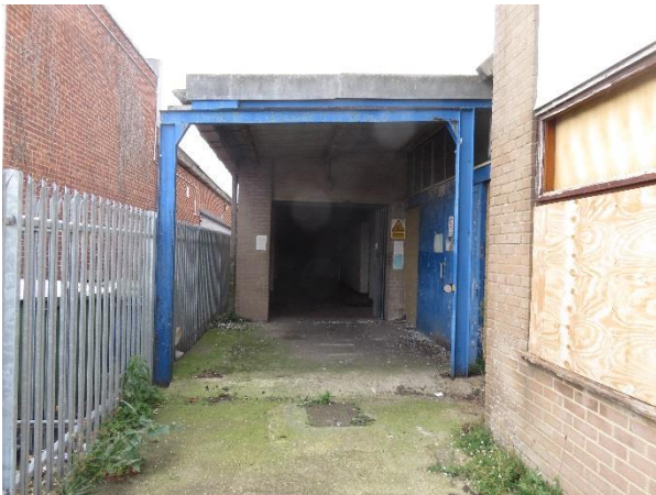
Southern Internal Access Point
