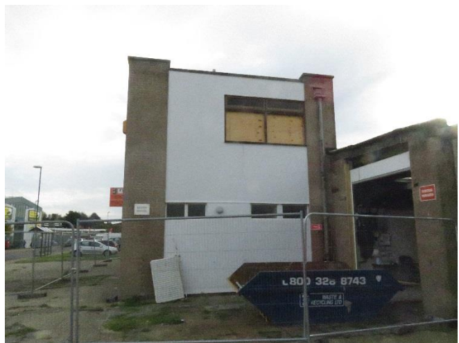
Northern Internal Access Point
