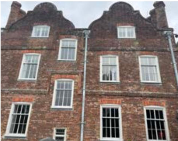
Image 9: Sash windows on the rear aspect of the property, which include potential gaps.
