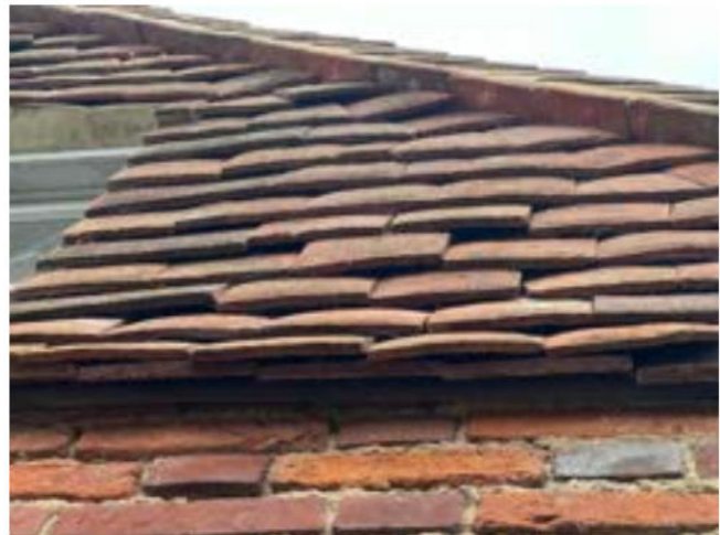
Image 10: Hanging tiles on one dormer on the main house. Note the gaps under many of the tiles.
