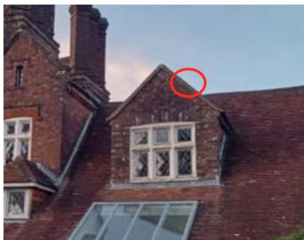
Image 21: Emergence location of the common pipistrelle beneath roof tiles on the eastern aspect.
