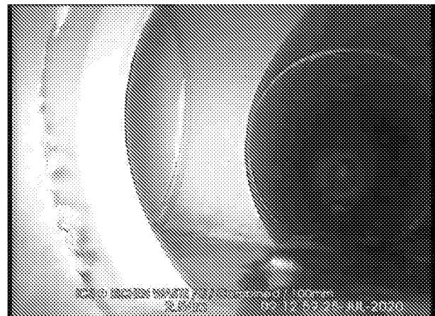
4, 00:02:02, 2.54 m Connection at 10 o'clock, 100mm diameter
