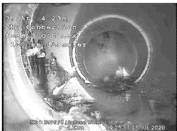
3, 00:01:19, 4.23 m Connection at 9 o'clock, 100mm diameter
