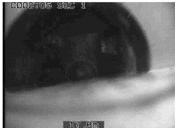
FW1X_ae57d161-f9c4-4092-a28d-53740de2bdf6_20180110_193636_768.jpg, 17.80m Finish node type, manhole, reference number: FW1 / NO
