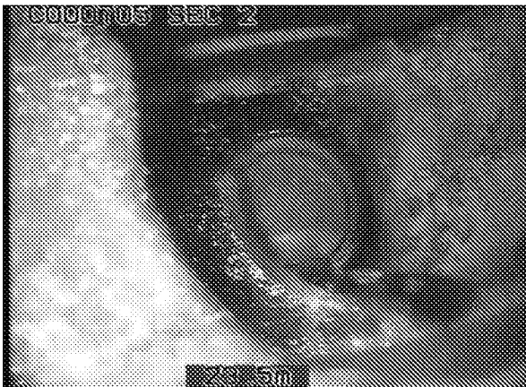
FW2X_123d7814-9d39-47bc-8a50-48c4b4c2e600_20180110 _194216_024.jpg, , 23.50m Finish node type, manhole, reference number: FW4
