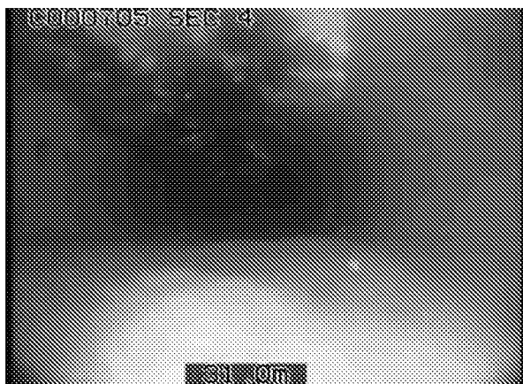
FW4X_d168865b-8a15-48a5-abc0-75b79300f2b4_20180110_200004_508.jpg, 00:08:06, 31.00m Attached deposits, grease at 12 o'clock, 5% cross-sectional
