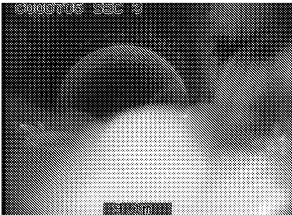
FW3X_87f3fb8b-06d2-4f23-9bf1-9e042a1563d5_20180110_194933_042.jpg, 00:00:00, 9.10m Finish node type, manhole, reference number: FW4
