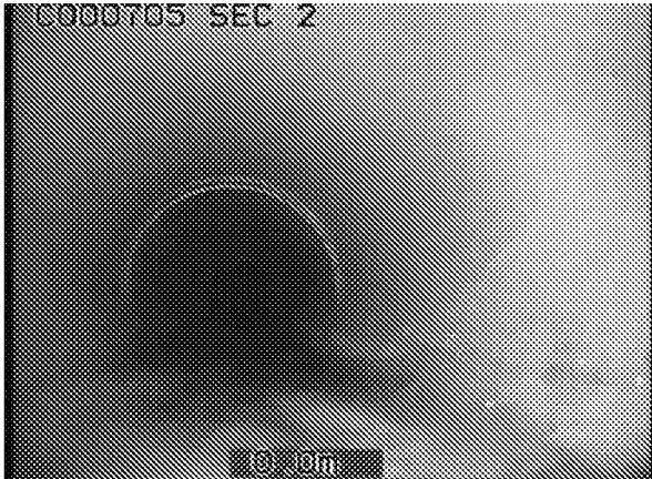
FW2X_3e2d9e45-481b-4e36-b275-d35d78e19be5_20180110_194004_497.jpg, 00:00:00, 0.00m Start node type, manhole, reference number: FW2
