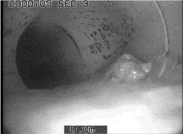
FW3X_ec21d8f3-e28e-4486-895b-98986cc3c2d7_20180110_194747_359.jpg, 00:00:00, 0.00m Start node type, manhole, reference number: FW3
