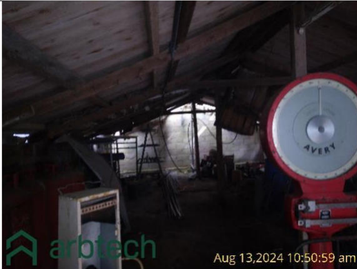
Figure 9- Hole back of roof of B3b
