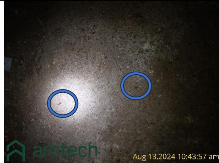
Figure 10- Droppings found on the floor of B3b
