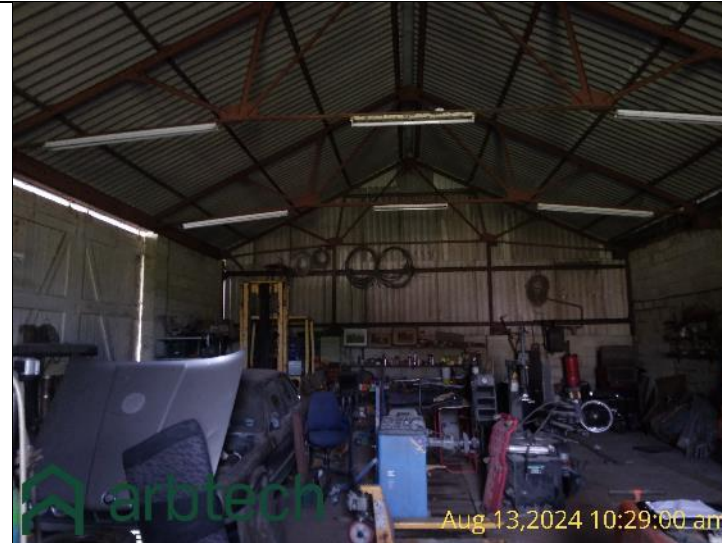
Figure 2- Inside of B1a
