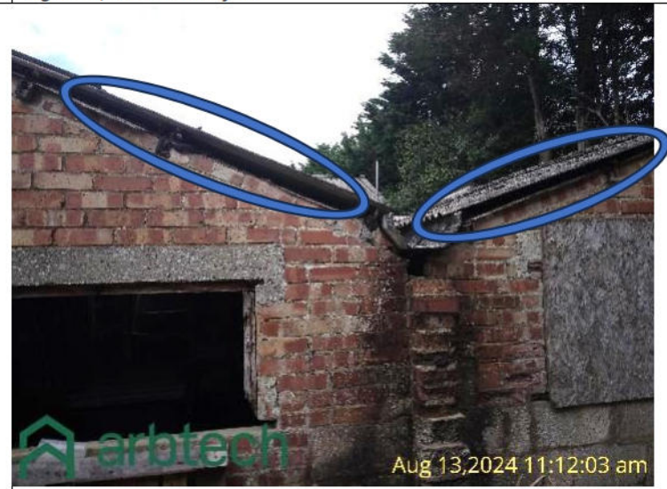
Figure 6- South view of B3a and B3b- Gaps between roof and gable wall circled.
