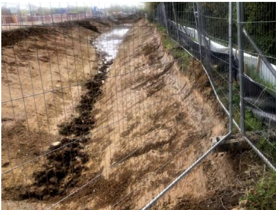
Photo 2 - Excavation of pond looking from west to east, note slope of southern bank too steep, corrected later with clay liner
