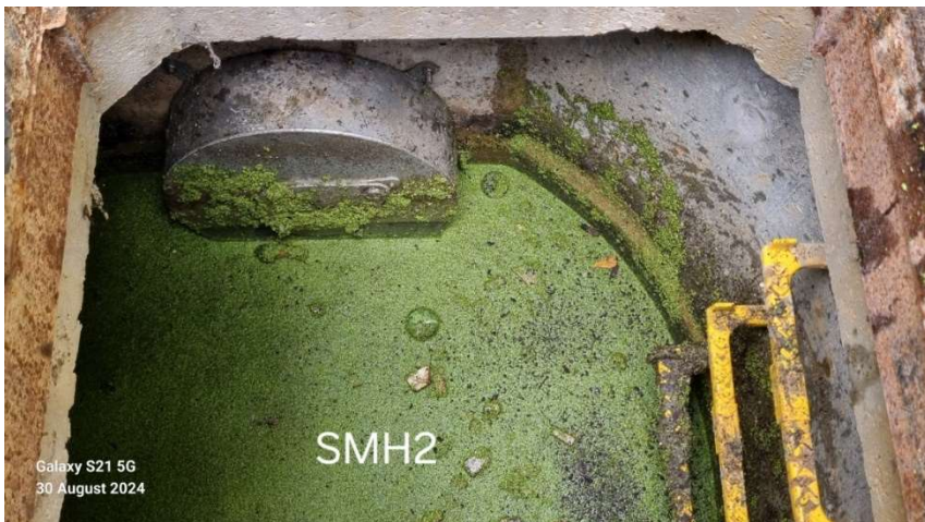
30-08-2024 SMH2 - Completed and in operation.
