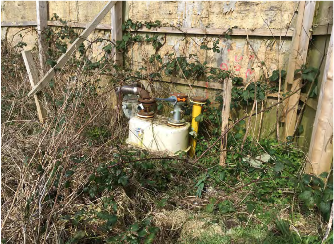
Photograph 5: Evidence of potential gas mains along the north-eastern boundary of the site. Now understood to be disconnected from the road.
