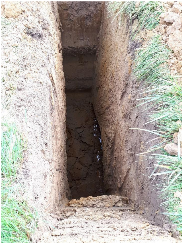
Plate 15: TP50 collapse and seepages
