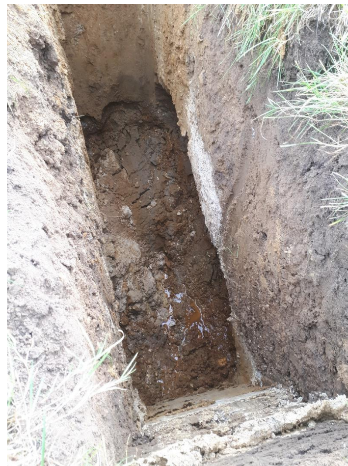
Plate 20: TP47a collapse and seepage
