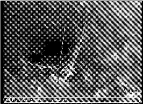
X_186b6554-4b67-40cc-a5d0-0c324681b8c7_20181025_200526_755.jpg, 00:00:30, 3.88 m Settled deposits, fine, 10% cross-sectional area loss
