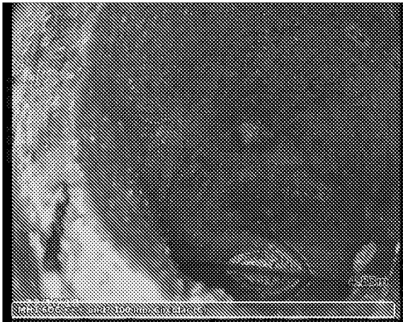
20181022-085911-snap0001.jpg, 00:00:40, 4.83 m Finish node type, gully, reference number: Gully
