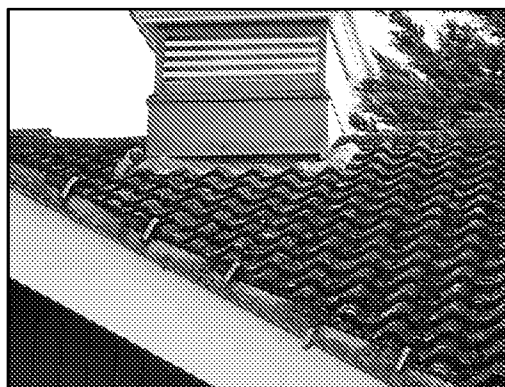
Figure 12 – gap under the base of the stalled tower
