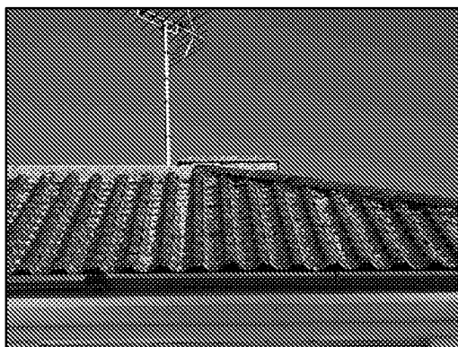
Figure 11 – gaps under hip tiles
