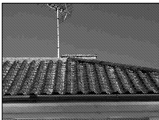
Figure 11 – gaps under hip tiles
