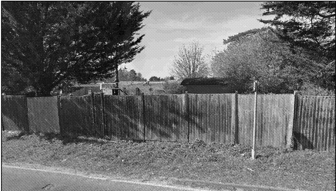
Figure 10 Gap in roadside screening 2
