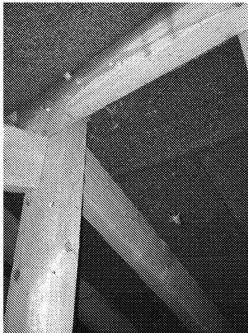
Photo 11: Loft void is lined with bitumen felt
