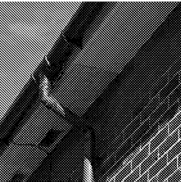
Black guttering and downpipes
