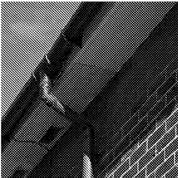
Black guttering and downpipes
