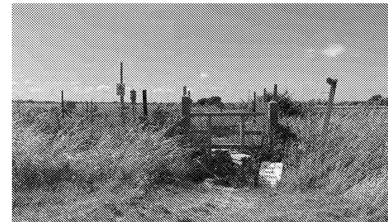
Pedestrian crossing on railway
