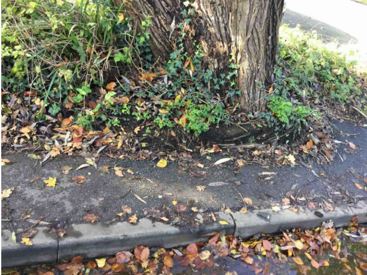
Photos of tree limiting width of footpath
