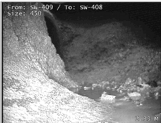
M/H NEEDS BENCHING
