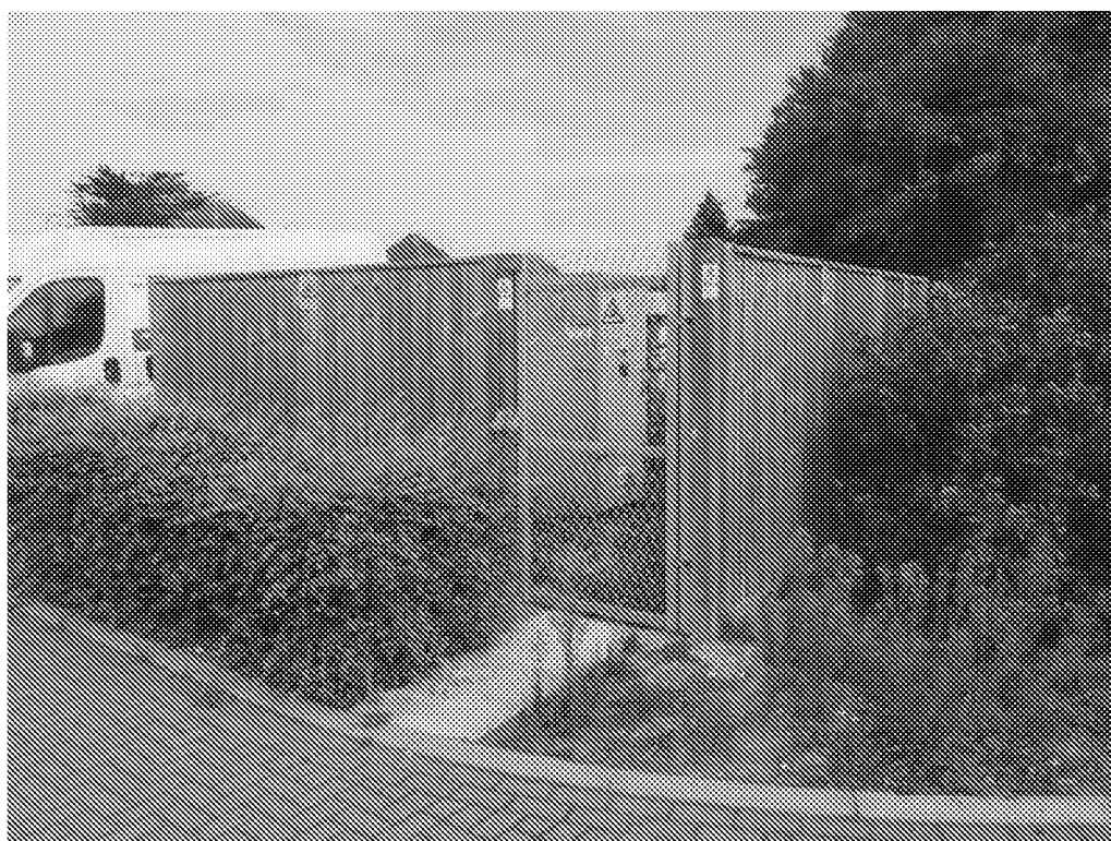
Electrical substation to the south of the site (facing north)
