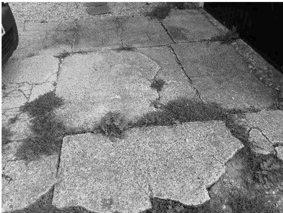
Broken slabs on driveway
