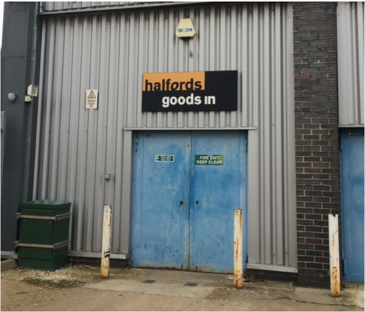
Existing 'Goods In' panel to be retained Clean only.
