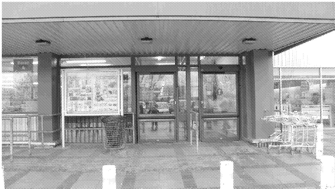
Entrance lobby to be replaced with larger unit with sliding doors
