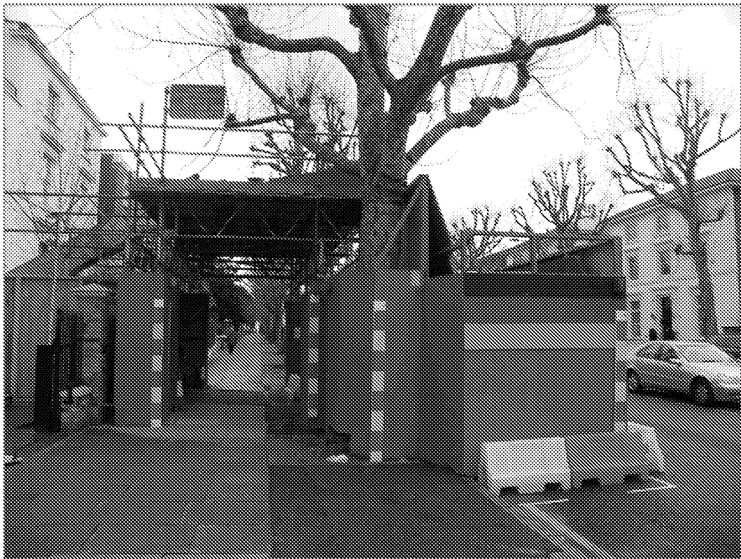
Picture 6: Where trees are off site, or public access is required through the work zone, boxing around the tree may be feasible.
