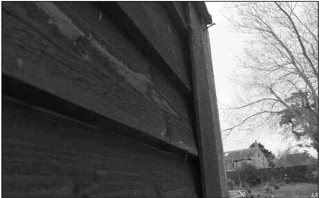
Photograph 8. Gaps created by a fascia board fitting to the caravan.
