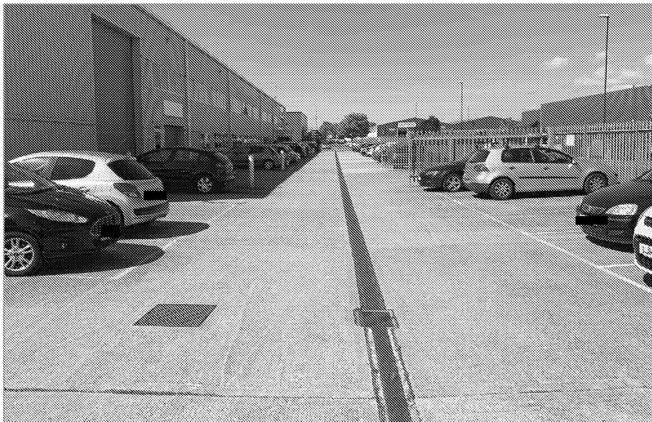
Figure 9: Car Park ACO Drain (Source: Unda Consulting Ltd)
