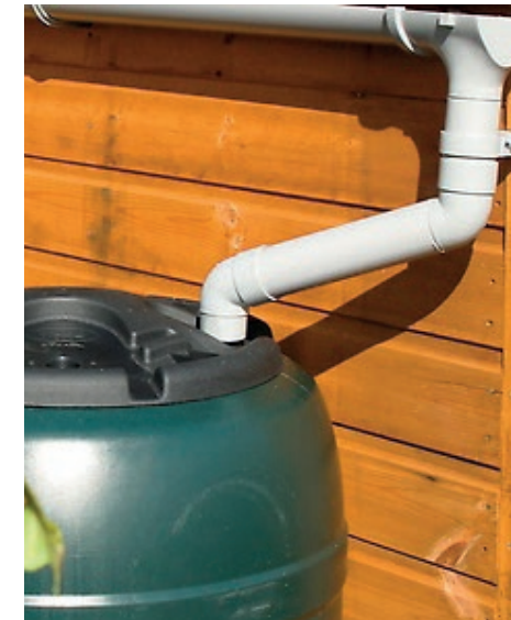
Rain water collection
