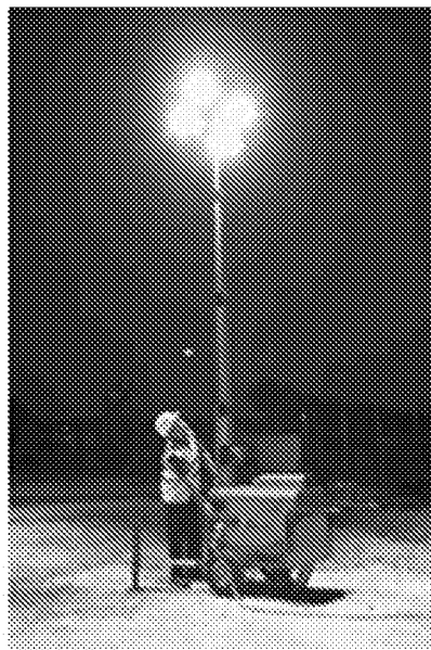
Typical Mobile Lighting Tower
