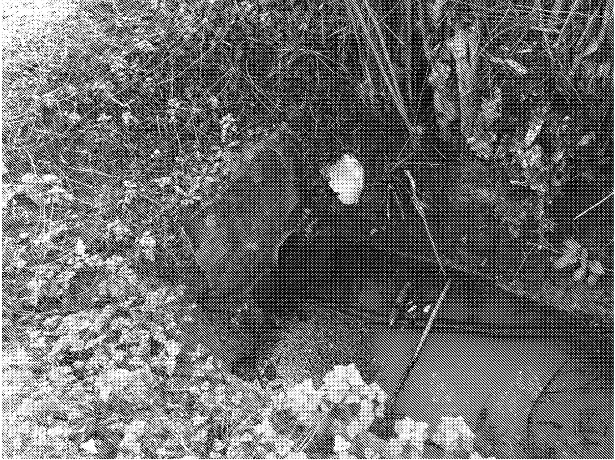
Pipe connection underneath Southern Water
