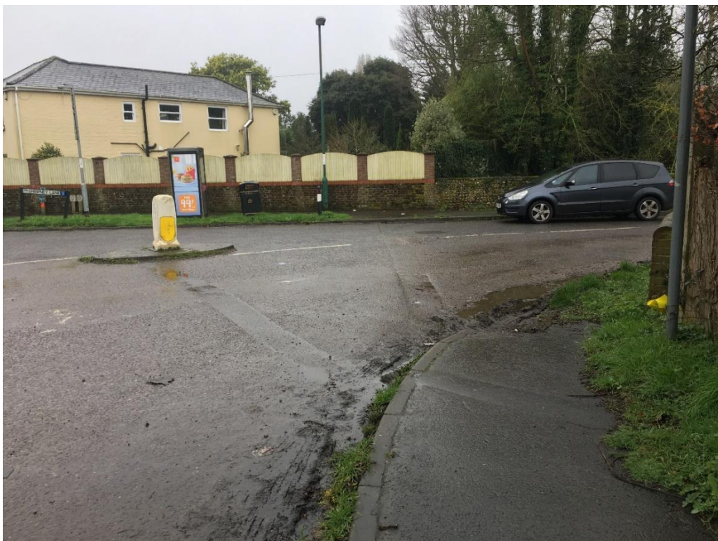
Photo 2.2 - Site observations suggest vehicles mounting the existing footway at the point where pedestrians will be encouraged to cross
