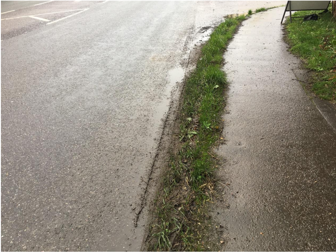
Photo 2.3 – Site observations indicate vehicles driving very close to the carriageway edge
