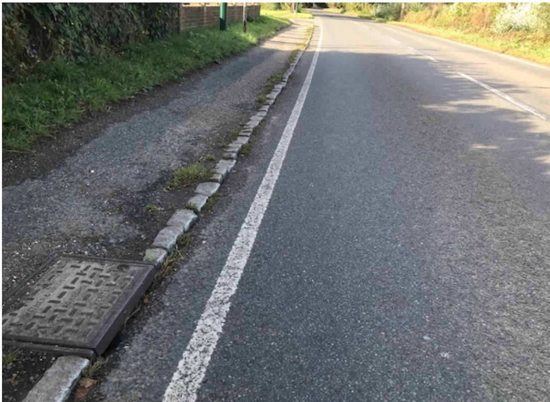
Photo 2.5 - Low upstand at the proposed west side crossing point allows vehicles to easily run over, which creates potential conflict between vehicles and pedestrians
