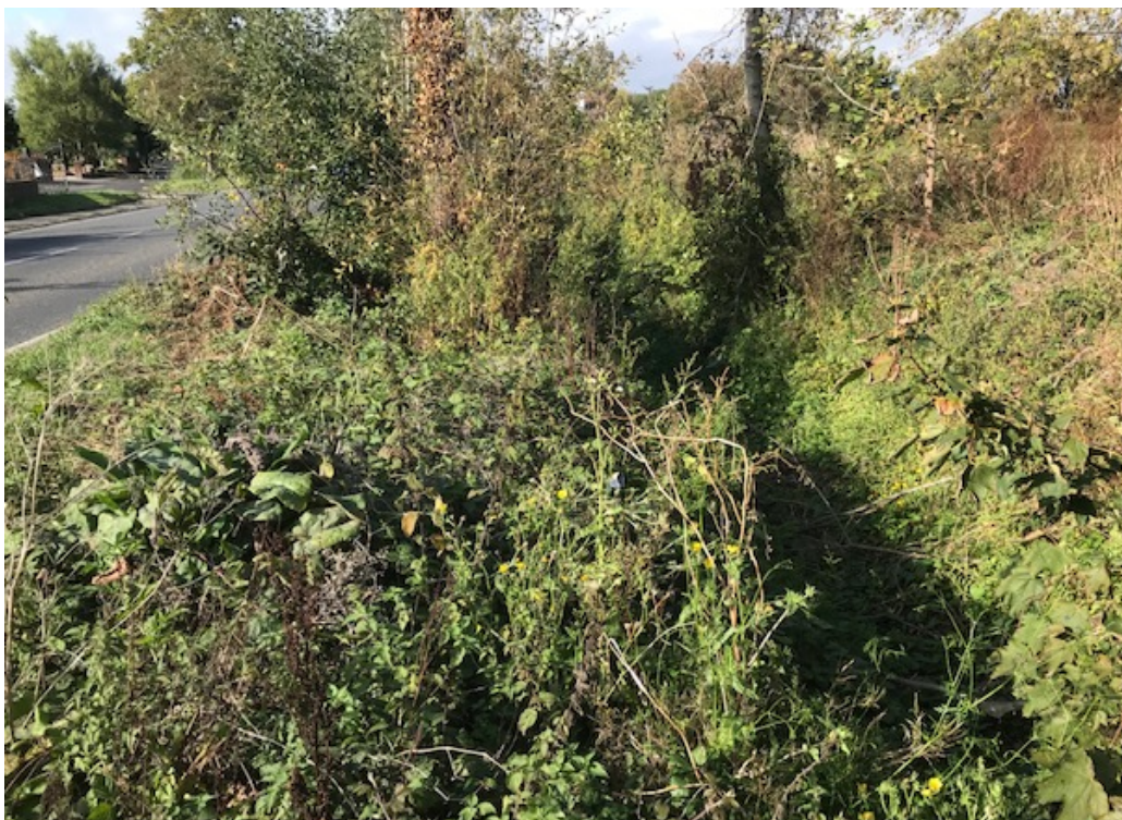
Photo 2.1b - Visibility to the north from the proposed junction. Also Problem 2.4 & Problem 2.8 - The ditch that is present will present a danger to footway users and increase severity of those involved in loss of control collisions.
