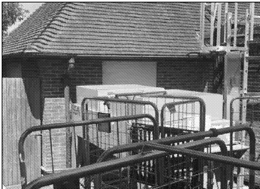
Figure 9. Two Rear Condensers and Roll Pallets/cages
