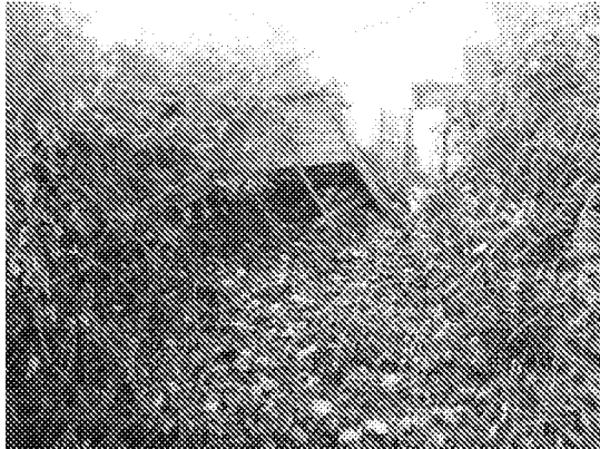
5. Dilapidated shed covered in bramble (TN3)
