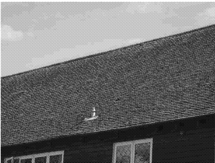
Building B1 - roof tile with gaps
