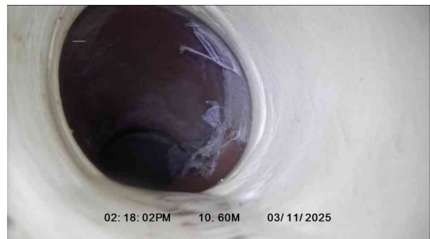
4, 00:00:35, 10.60 m Point repair, localised lining from 12 o'clock to 11 o'clock
