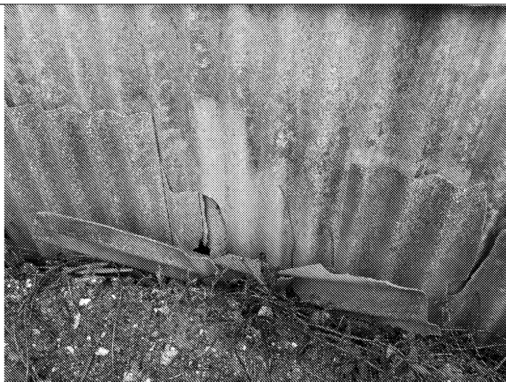
Damaged asbestos cement sheeting at the rear of the workshop.
