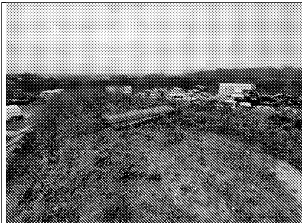
Asbestos cement sheeting on northern bund (near MTP332).
