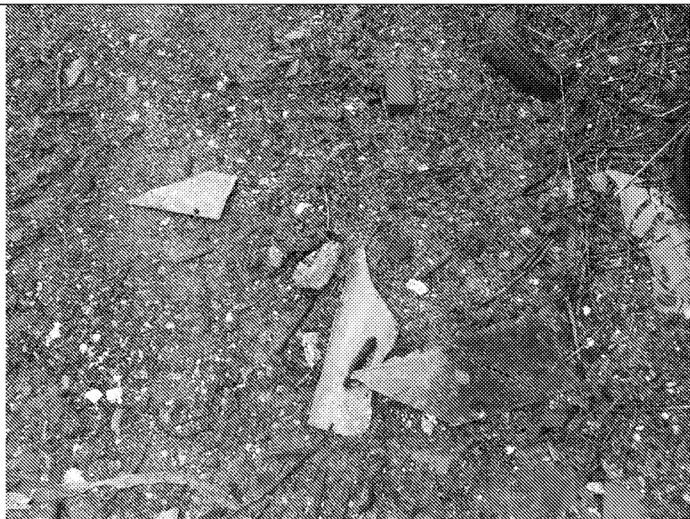
Damaged asbestos cement identified on the surface behind workshop.
