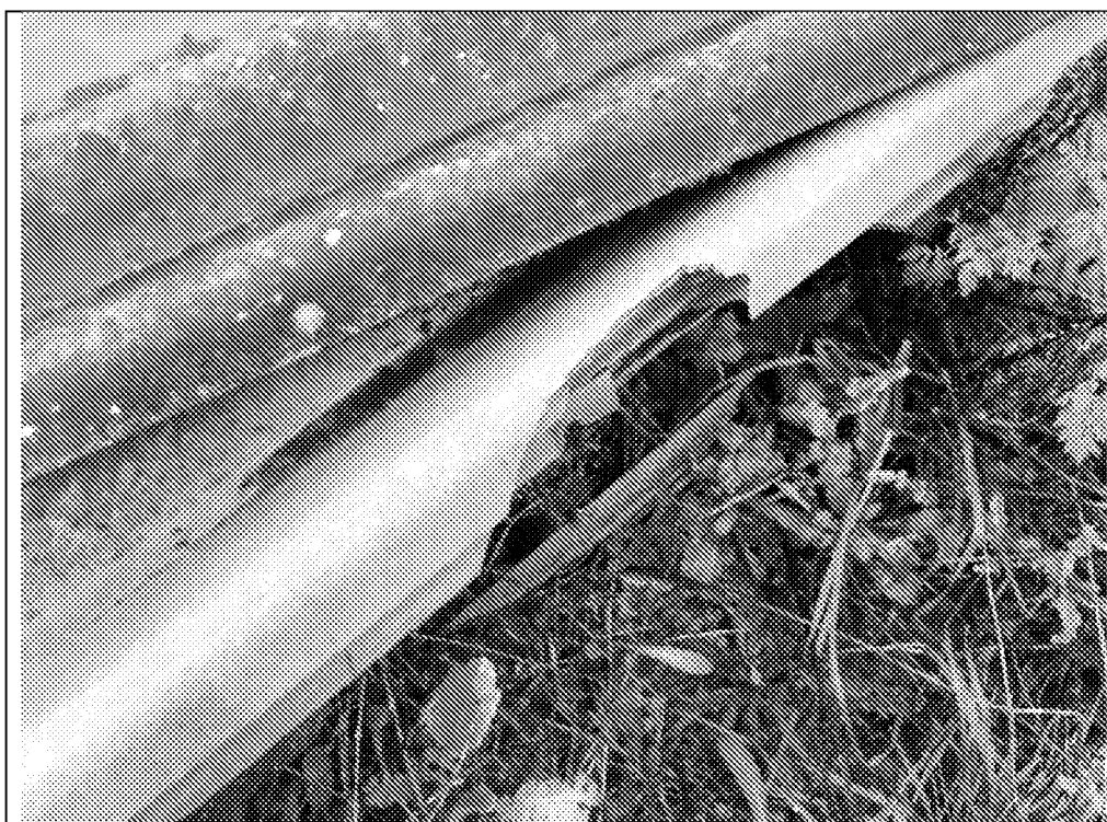
Asbestos cement sheeting damaged on northern bund (near MTP332).
