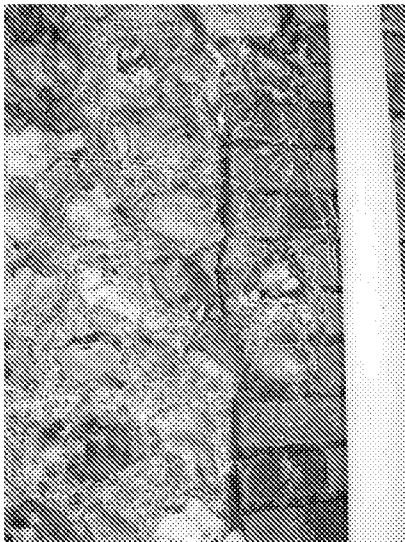
Crack in wall, south east corner
