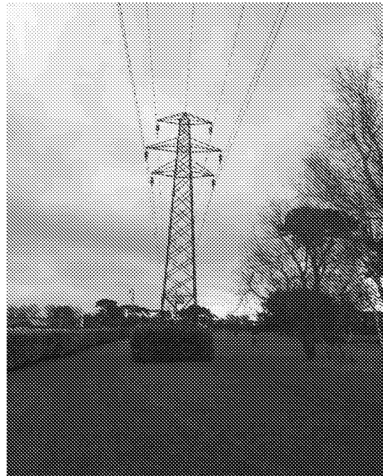
10. Overhead Power Lines and Pylon
