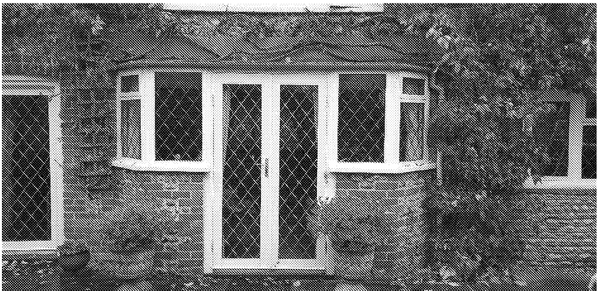
Photograph showing the rear bay window. The lead roof is proposed to be replaced as it currently falls the wrong way towards the house. See Note 07 on drawing 19068 2.01.
