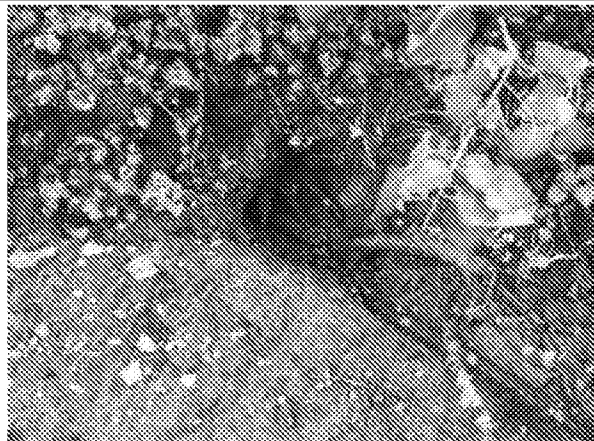
Photograph 15 Blocked hole (southern boundary).
