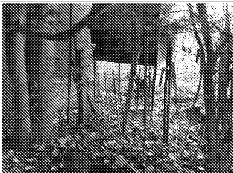
Above ground storage tank observed adjacent to northeast of site.
