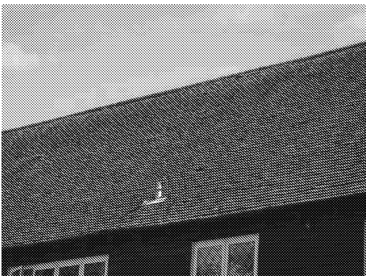
Building B1 - roof tile with gaps
