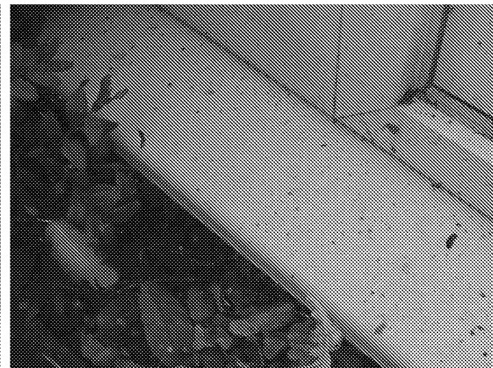
Bat droppings - building B1
